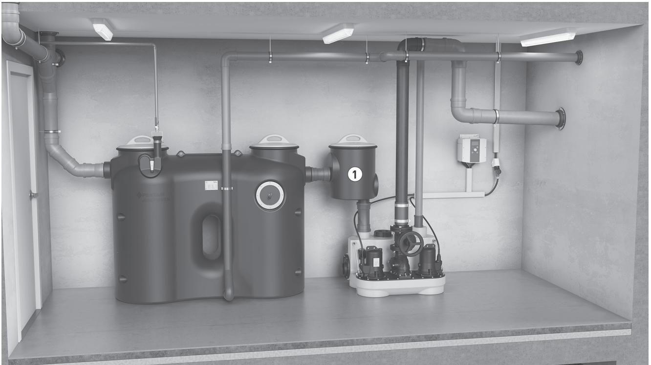
Example of installed Splitfix with sampling tank
